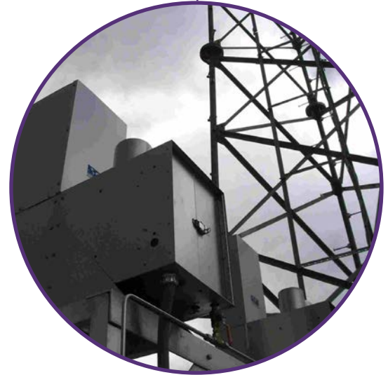
Telecommunications 150 watt system remote radio repeater tower, USA
