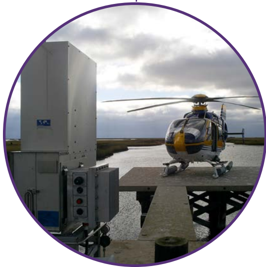
100 watt system cathodic protection, Louisiana, USA
